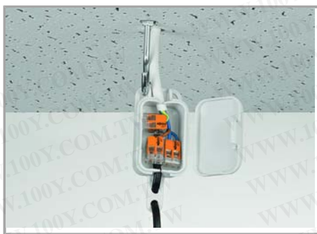
Pendant light connection in suspended ceilings
