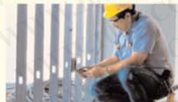
COOPER Wiring Devices
